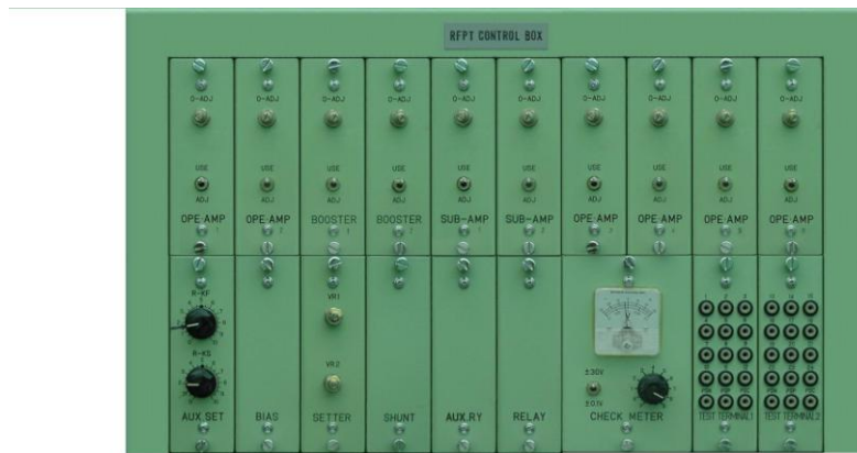
Figure 25. Instrumentation modules for the nuclear power plant of Laguna Verde that were designed and built at ININ. They are in the electro-hydraulic control system for the turbo pumps.
